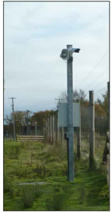
Precedent CCTV Mast
